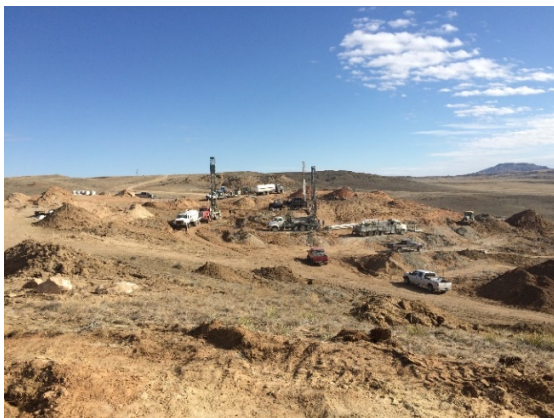
Nichols Ranch ISR Project, Header House 6 Facing North, March 2015
